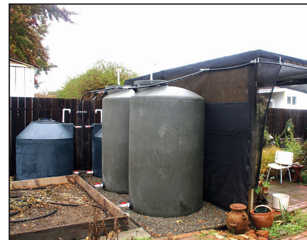
A rainwater catchment system can include multiple large tanks.
