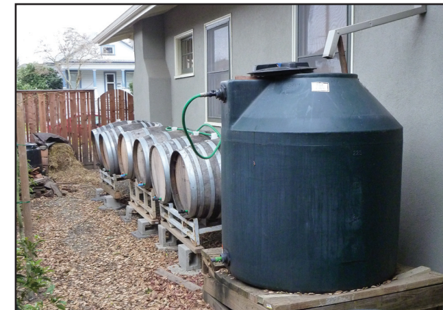
A local rainwater catchment system that utilizes old wine barrels.
